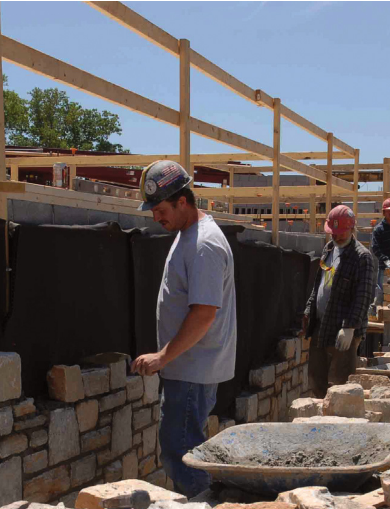
Members Building BAC's Future: John J. Flynn BAC/IMI International Training Center under construction
